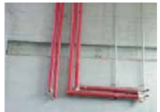
Asbestos lagging on pipes
