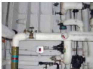
Asbestos insulation on pipes
